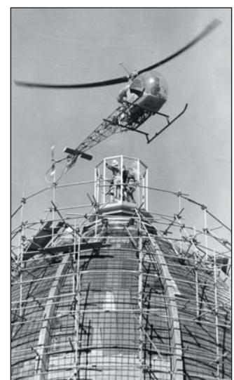
A helicopter installs the lantern in the dome of the Bahá'í Temple in 1961
